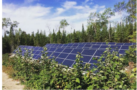
An array of solar panels at Falcon Trails resort
